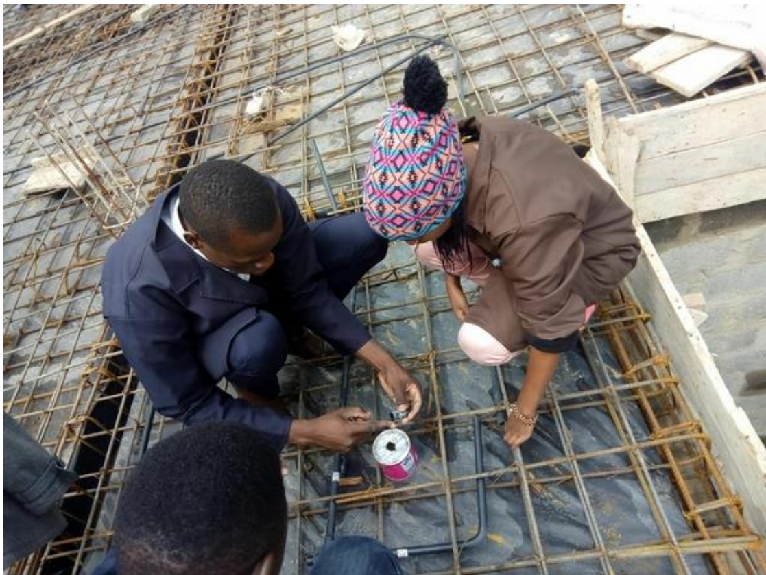
Gaining 'hard' technical skills: CAP YEI Students practicing wiring at a construction site near Nairobi. Employers insist that, in training workers, soft skills are just as important as technical skills.
